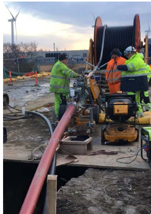
Fig. 3: Installation of a single cable phase in a single duct with the Watucab technology
