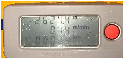
Fig. 6: Monitoring of the installed cable length and installation speed during the installation of a 3200-meter-long cable
