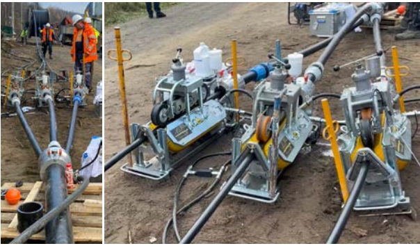
Fig. 4: Installation of 3 single cable phases simultaneously in 1 duct, a special adapter with three inlets installed on the duct (left). The three cable pushers are synchronized with each other to install with equal speed the three (right).
