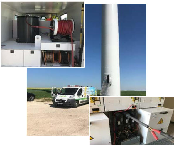
Fig. 11: Test setup with the DAC system mounted in a test van and connected to the 30 kV T-conductor termination by a test adapter.
